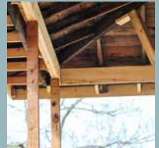
March 2019 – Front porch work complete with new beams installed to reinforce existing structure!
