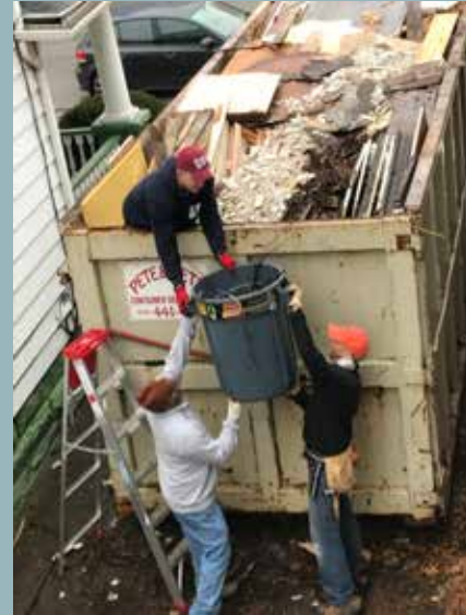
November 2017 – Volunteer work team assists with demolition inside and an old garage outside!
